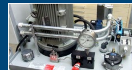
Hydraulikaggregat Power unit
